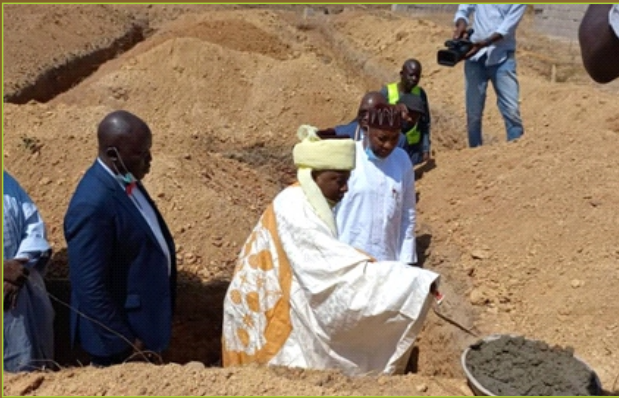
→ Representative of Emir of Bauchi officially laying the foundation of "The CIBN Bankers Hall"
